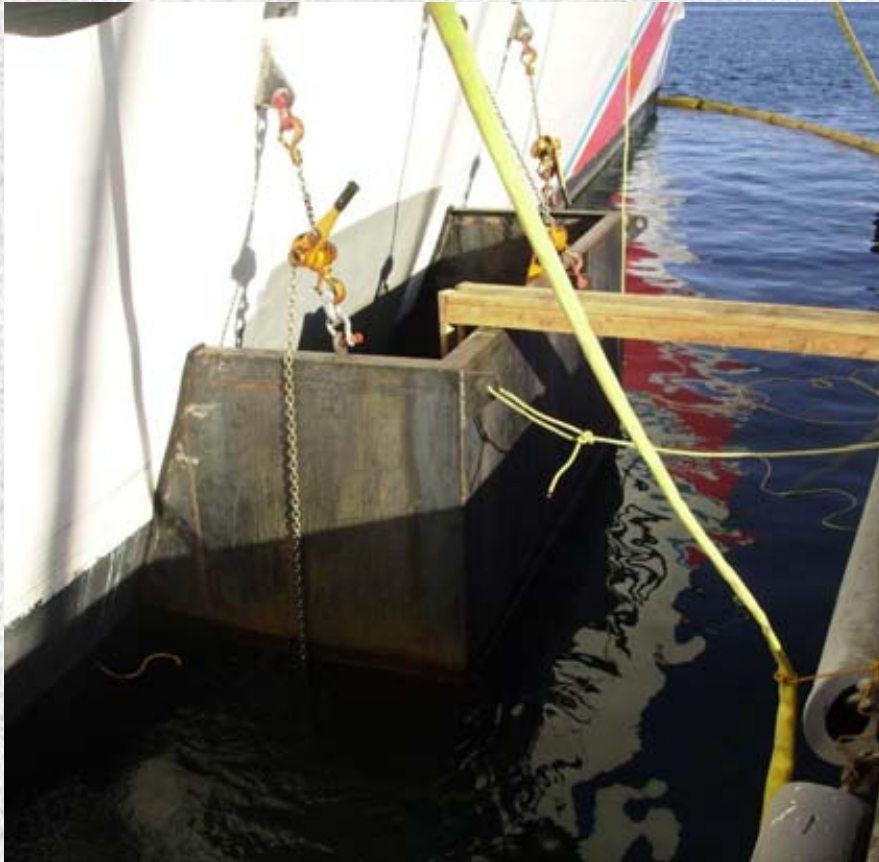
Installed – Ready for Work
